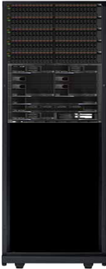
Rack with External Storage
